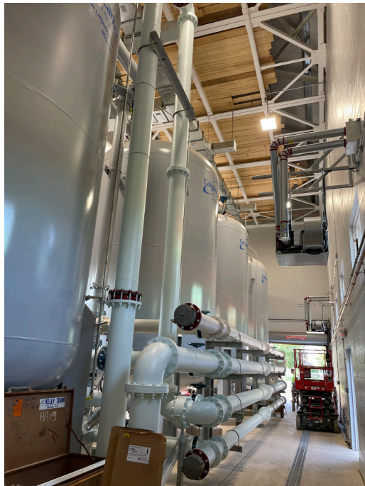
Willingboro Well 5A Water Treatment Plant (granular activated carbon). Photo courtesy of Willingboro Municipal Utilities Authority
