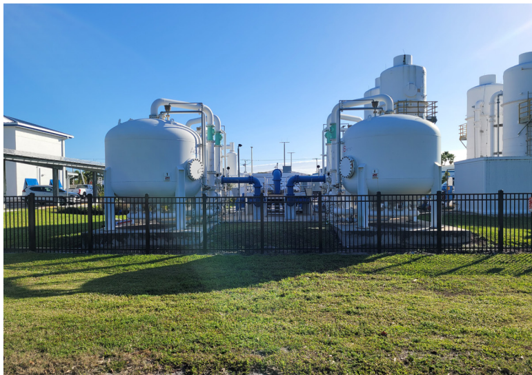
City of Stuart Water Treatment Plant (ion exchange). Photo credit: City of Stuart
