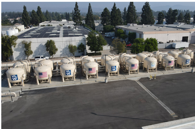
J. Wayne Miller, PhD Water Treatment Plant (ion exchange). Photo credit: Yorba Linda Water District
