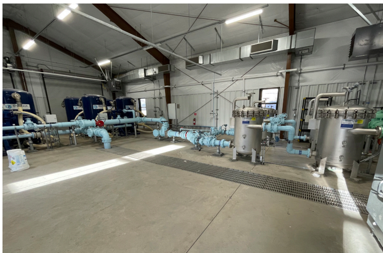
Stratmoor Hills Central Water Treatment Plant (ion exchange). Photo credit: Stratmoor Hills Water and Sanitation Districts
