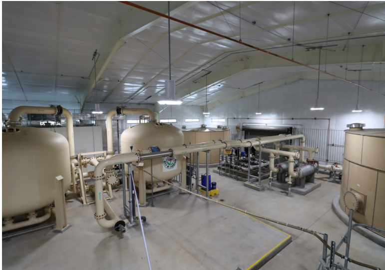
Aga Park ion exchange treatment facility. Photo credit: City of Fountain, Colo.
